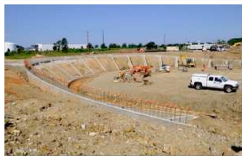
Melissa Cherry, mcherry@heraldonline.com -- The Giordana Velodrome is under construction as part of the Riverwalk development in Rock Hill. City officials hope to open the cycle racing track on Jan. 1.
